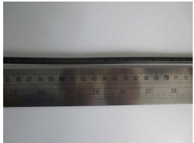
Cable(PV-F, 1 x 4.0mm 2 )
