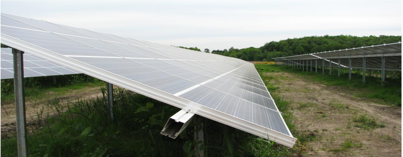
2MW Ground-mounted PV Plant in Guntramsdorf, Austria
