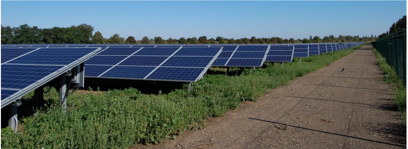
6.3MW Ground-mounted PV Plant in Rooksbridge, UK
