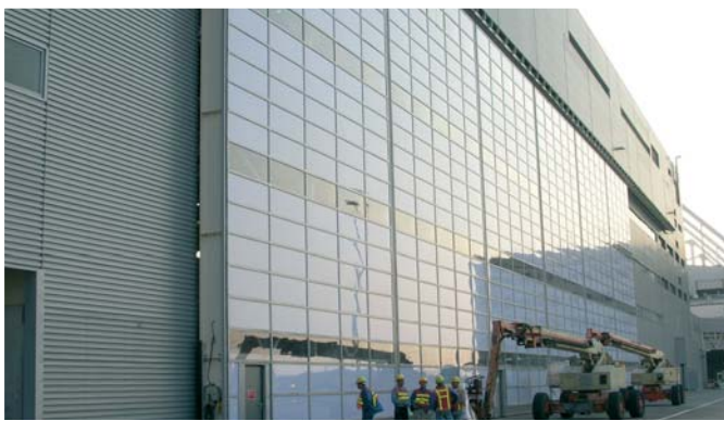
HAECO Hanger No. 2, Hong-Kong International Airport (Curtain Wall) 12.7mm Clear & Opal PALSUN® flat solid polycarbonate
