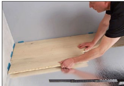
Start the next row from the left again. Simply click the planks together lengthways. Gluing the planks is not necessary.
