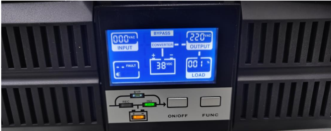
Figure _80 UPS operation panel
