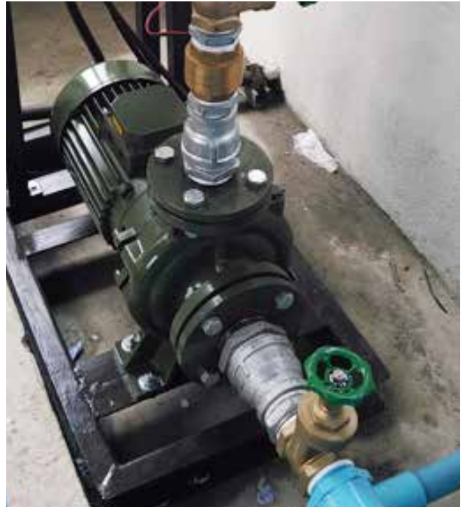
NR. 1 IR 50-160B THAILAND WATER SUPPLY IN A HOTEL
