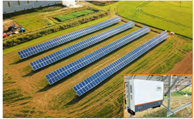
Lincolnshire, UK 140kW
