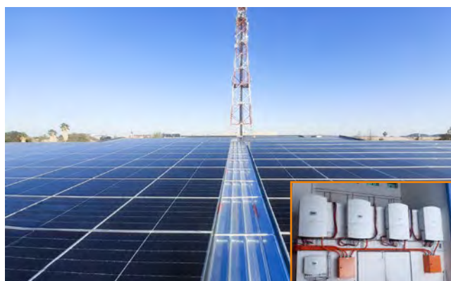
SolWorx Project, Namibia 272kW
