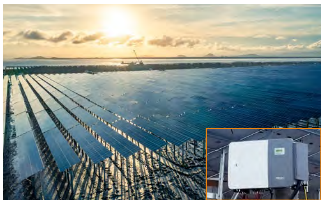
Zhejiang Ningbo Tidal Flat Project 300MW
