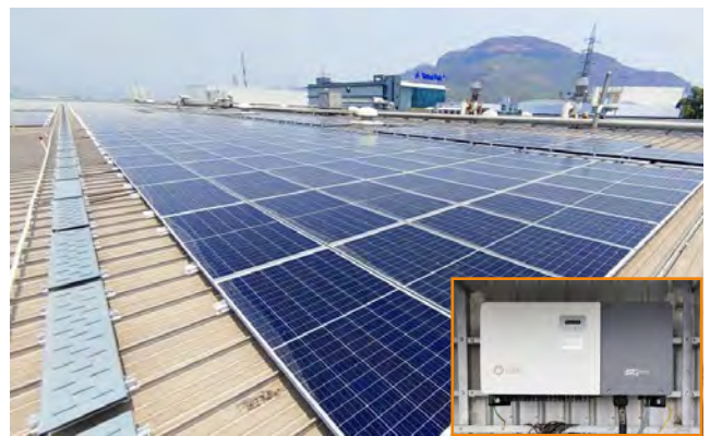
Tetra Pak Project, India 1MW
