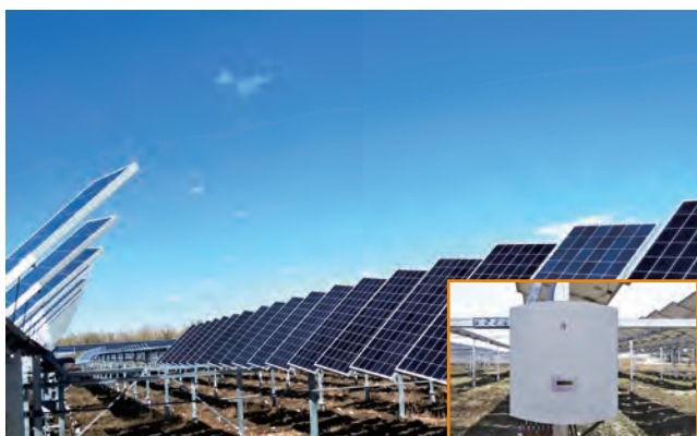
Hebei Zhangbei Agricultural-photovoltaic hybrid PV plant 50MW
