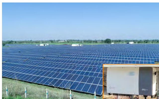
Soleos Energy Project, India 2MW
