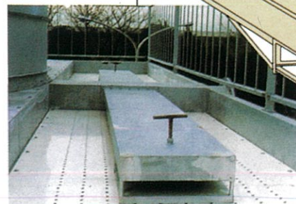
● Upper water tank and sprinkle equipment Double use of structure materials for upper water tank and sprinkle equipment makes the tower lighter with high efficiency.
