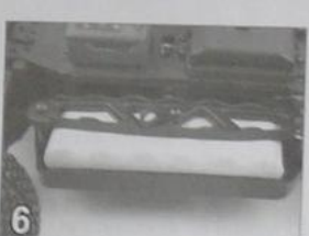
cover the battery box
