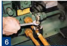
6 screw the valve to the right until it stops then screw it to the left
