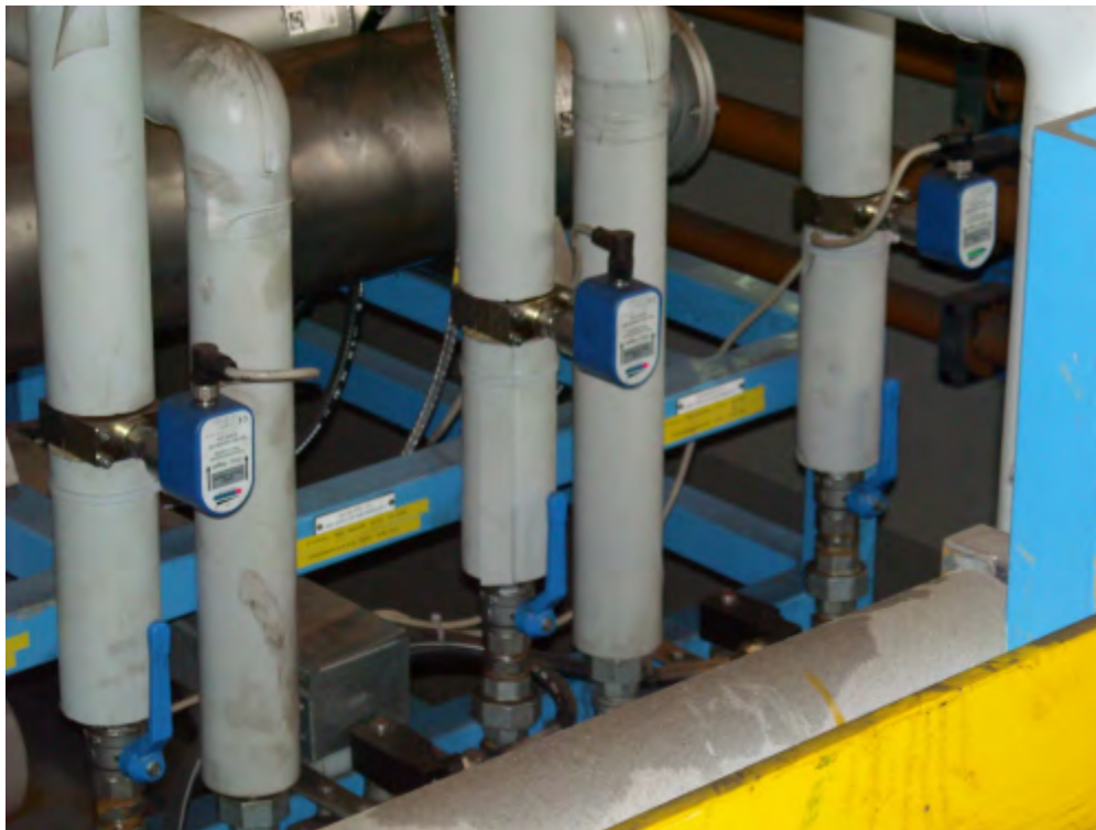
Picture 4: Control of a lubrication oil line with flow rate sensors and Serv-Clip -2 at a continuous pickling line.
