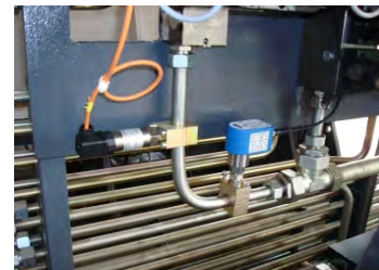
Picture 2: Pipe measuring point Serv-Clip -1 with pressure sensor (threaded coupling G 1/4")
