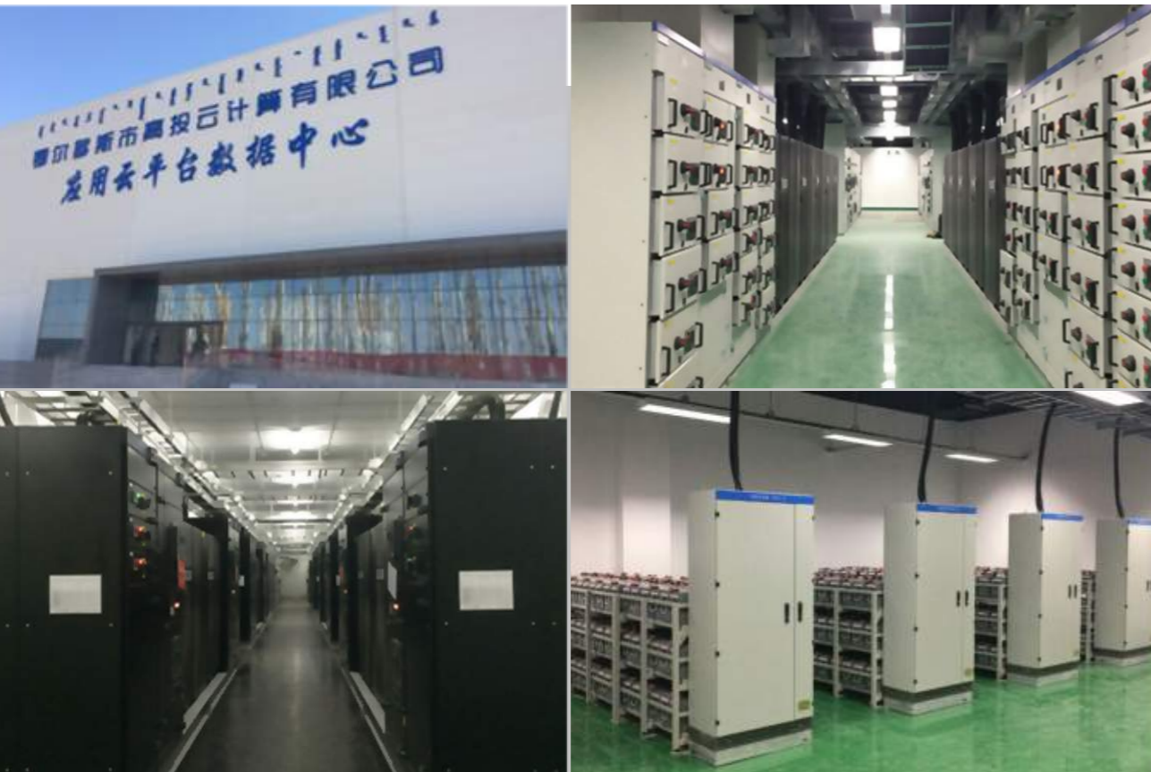
Amazon West Cloud Valley Data Center in Ningxia
