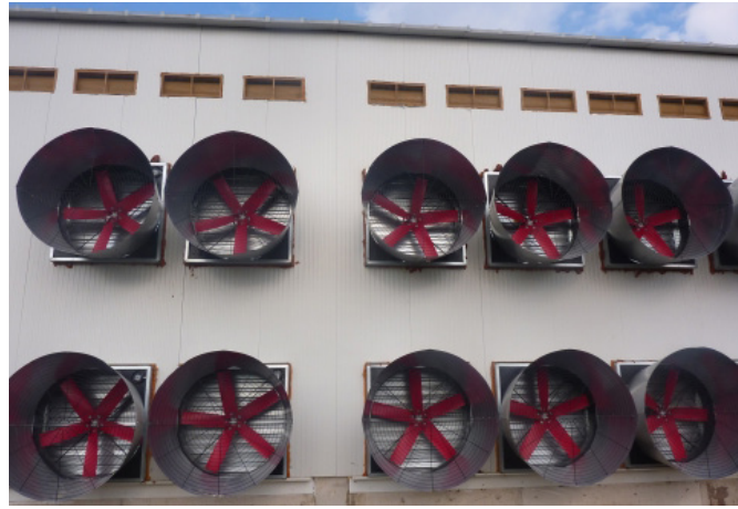
Ventilation applied in poultry houses in the Middle East
