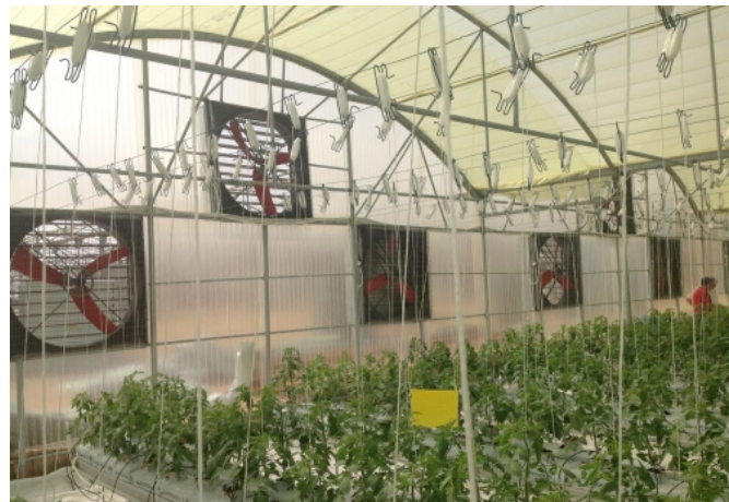
Fans applied in a tomato greenhouse in the Middle East
