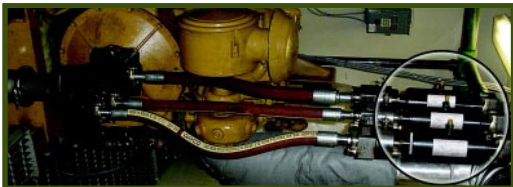
The original thinking on this installation was that the hoses would dampen the noise and vibrations. When that failed these three Suppressors were installed and the system was quieted.
