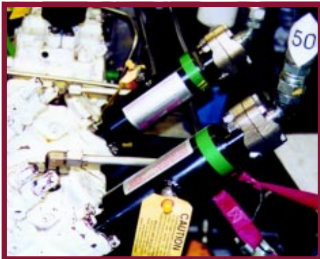
Pictured are two variable displacement pumps that operate at 1800 rpm. The combination of two pumps operating at a high speed made this a noisy application until the two flange mounted Suppressors, identified by the green bands, were added to the pump outlets.
