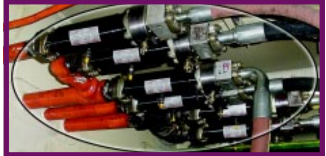
These six Suppressors quieted multiple flow lines installed in an overhead configuration.
