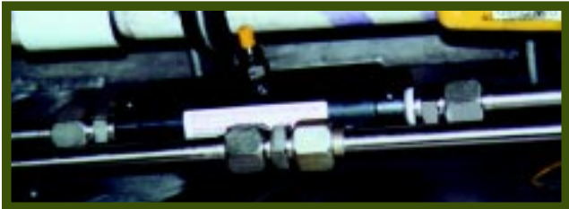
The straight thread suppressor is easily added to a run of tubing. There were two tube joints at this location. One was easily replaced with a suppressor.
