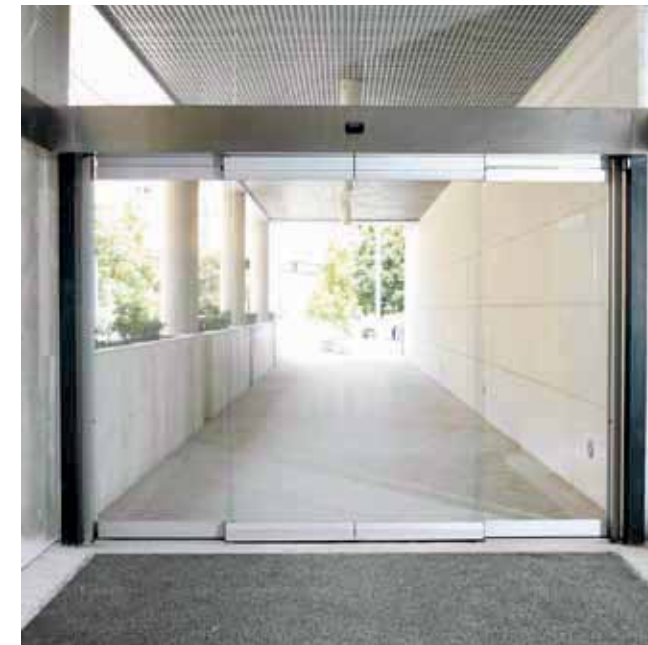
Panic break-out door without vertical stiles. Shopping centre.
